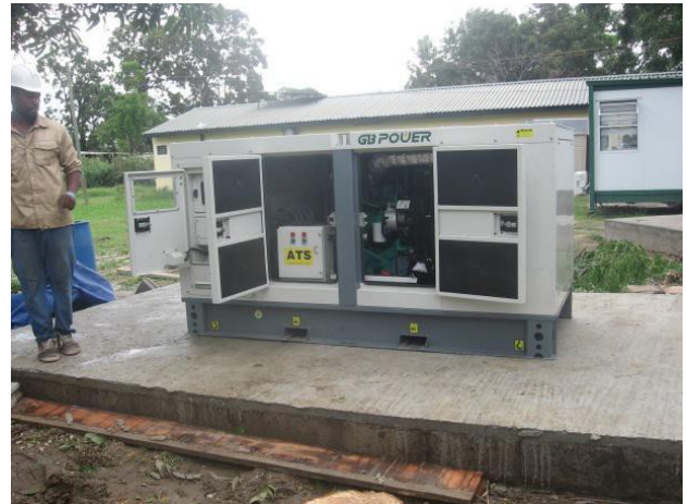
The new 60KVA generator in Lusaka, Zambia
