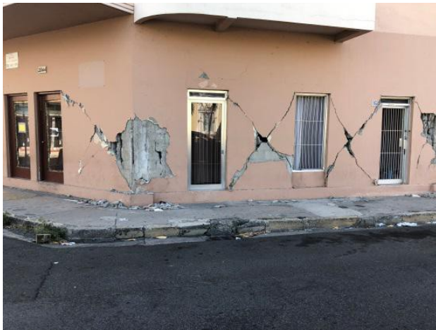
More earthquake damage to buildings in Puerto Rico.
