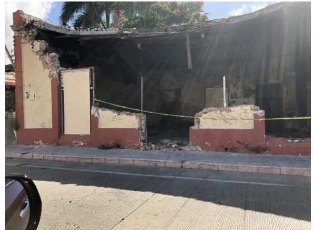
Earthquake damage to buildings in Puerto Rico.
